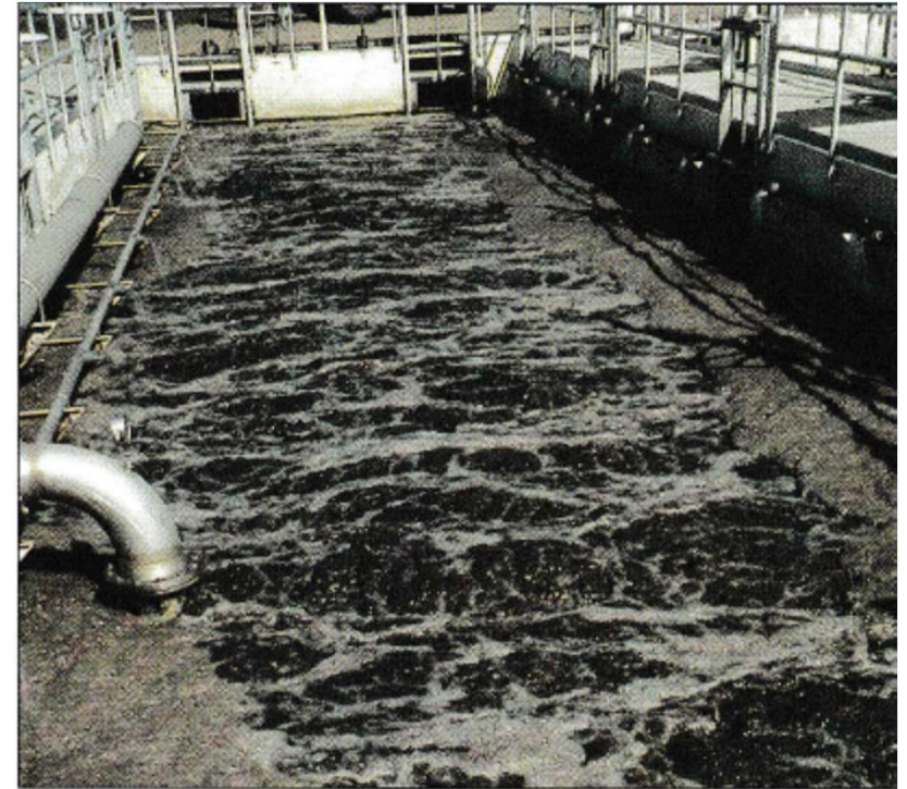
(b) An aeration tank. Note surface is frothing from aeration.
