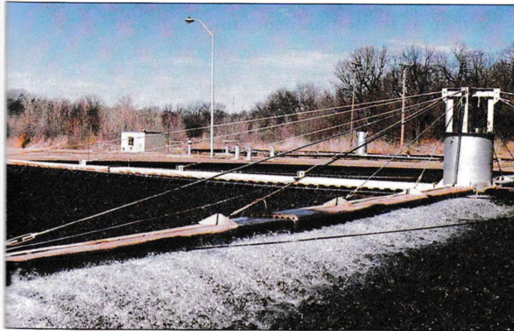
(a) Rotating spray arm of a trickling filter system
